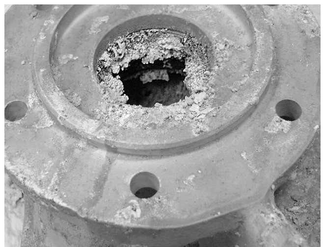
Figure 3-24. Magnesium Corrosion Products
